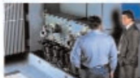
COOPER Power Systems
